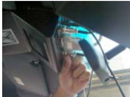
View of DB-25, interface, LED, camera and power cables being connected to control head.
